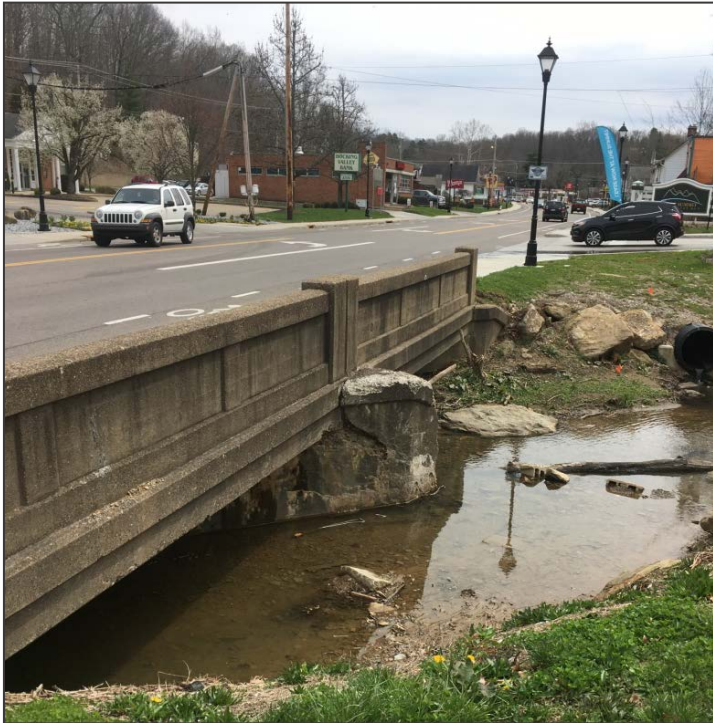
Existing Structure between Greenbrier Drive and the Richland Avenue entrance to the Summit at Coates Run
